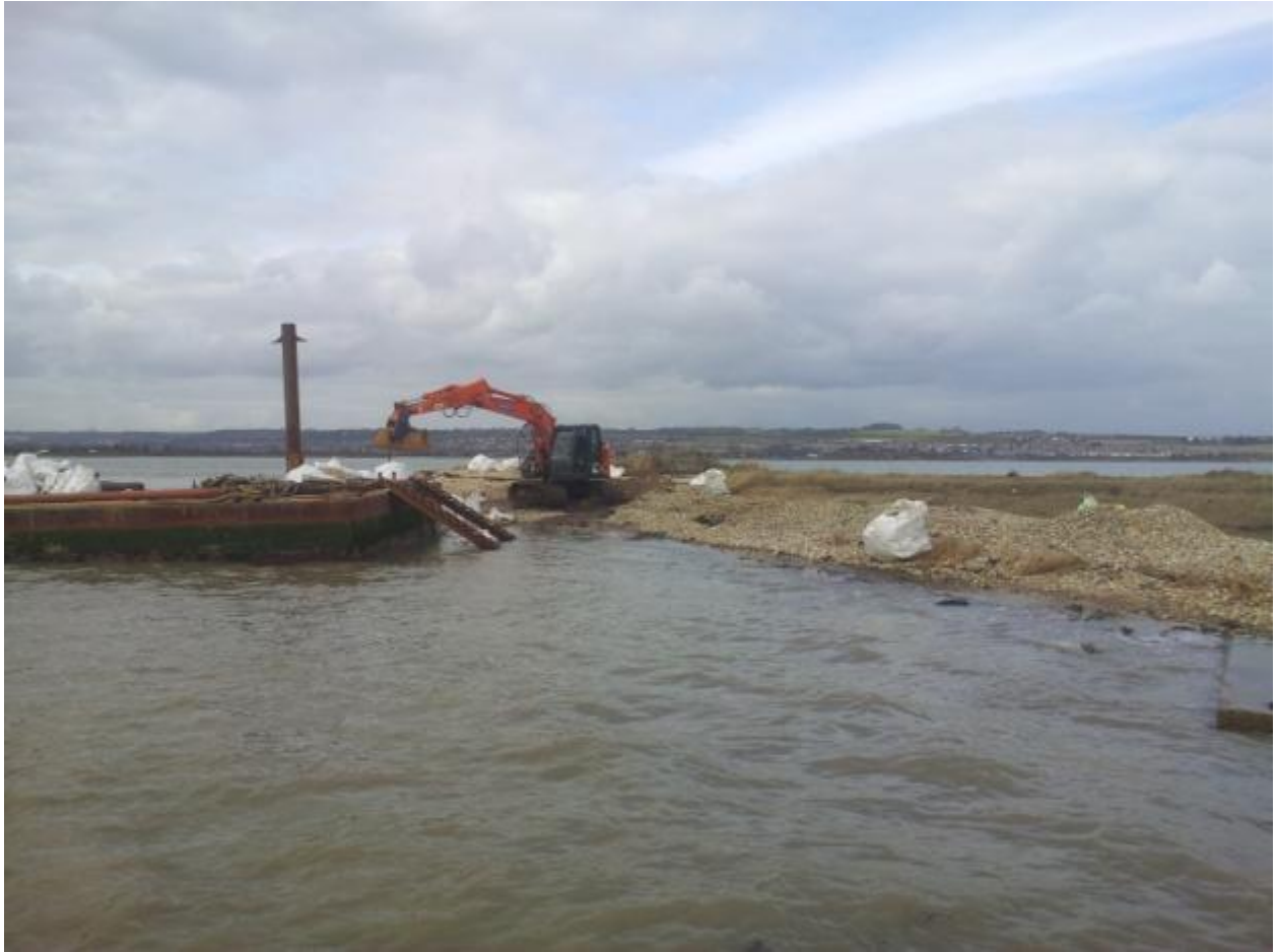
Figure 7. Excavator in the process of placing shingle bags within permissible parameters on Bakers Island, 2014.
